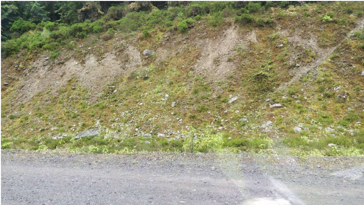
Figure 6-7: Exposed overburden cut with evidence of erosion/shallow slips (ITM 519555E, 583500N)
